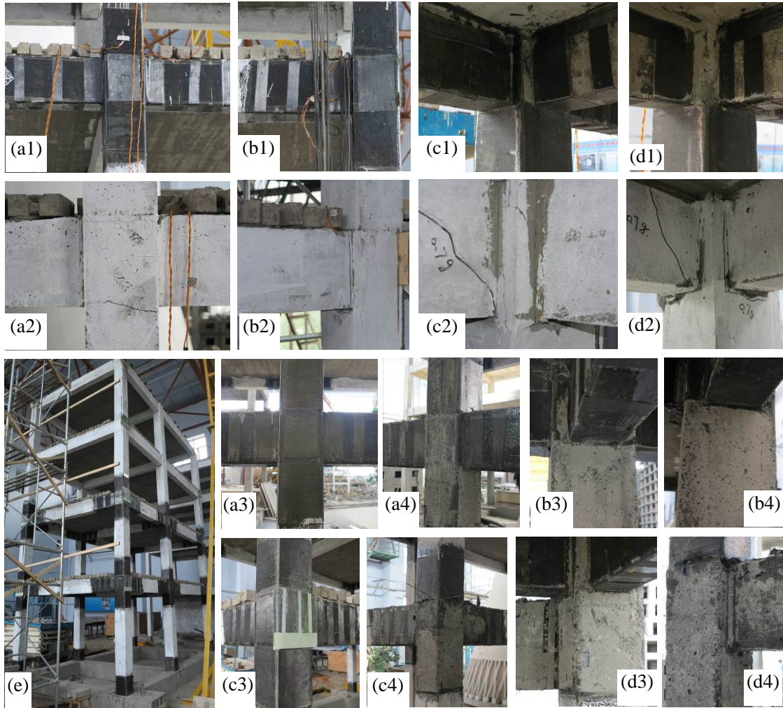
Figure 4. Failure modes of CFRP retrofitted RC frame model
